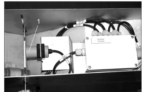
Figure 4 1 Limit switch for roof drier safety bracket
